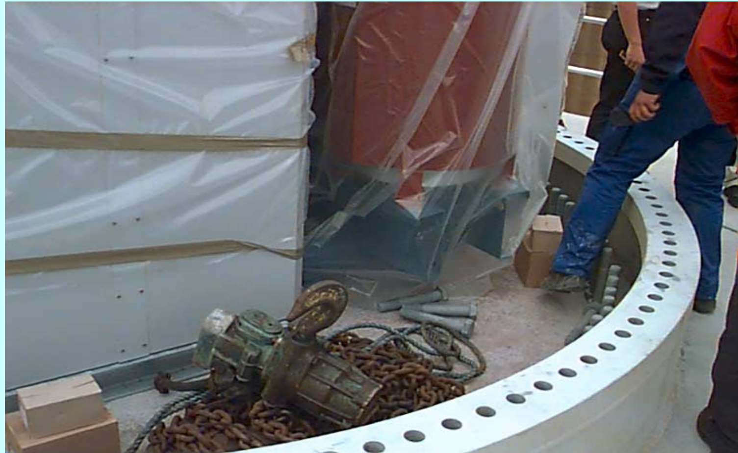
The 690V/30kV transformer of the dry type (without oil)
